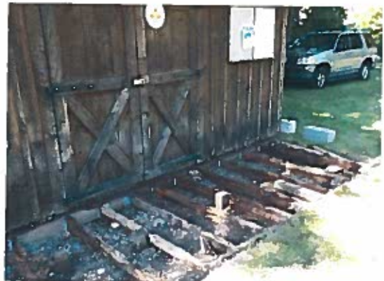
When we removed the decking, we found rotted wood and short 4x4s that were not secured to the ground or other boards.
