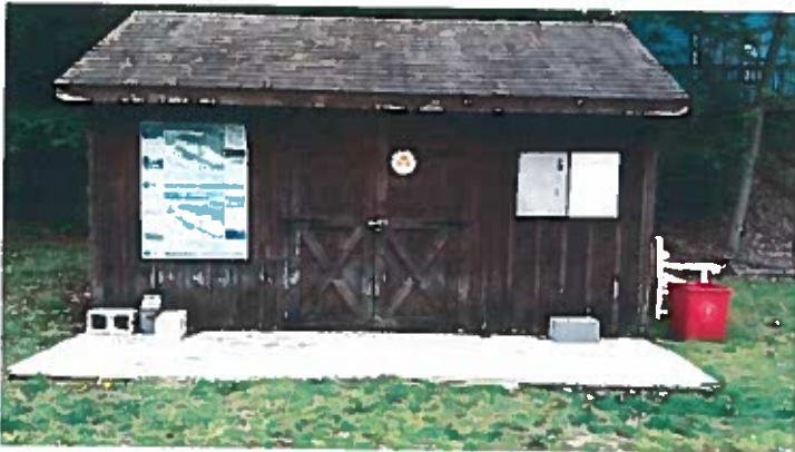
The existing porch consisted of warped Trex board.
